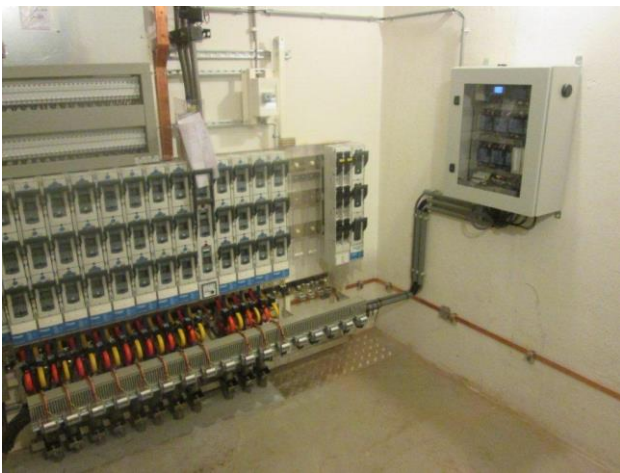
Fig 6 : Low voltage switchgear and measurement cabinet
